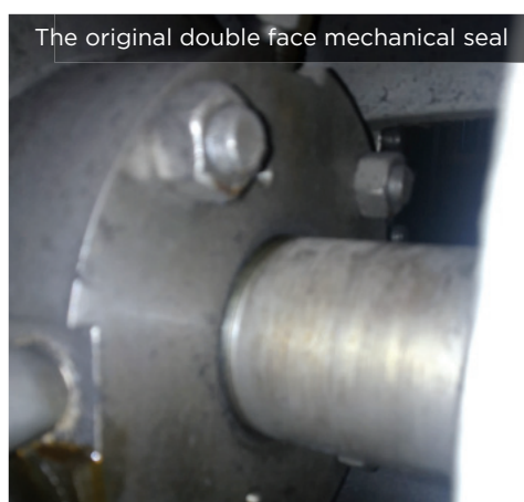
The information on the original pump
